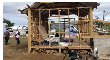
Demonstration houses built to show villagers how to build back safer Credit: Red Cross
