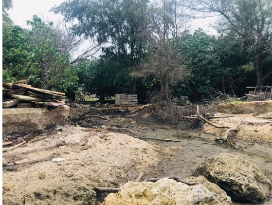
Part of the revetment which collapsed during the tsunami. (Photo courtesy of Manu Manuofetoa)
