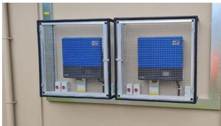
- Figure 14. Example of a metallic cage that protects outdoor inverters from theft.
