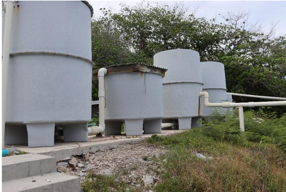
NFMRA Aquaculture Holding Facility Bio-filters and overhead water tanks
