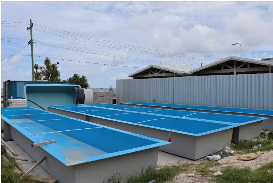
NFMRA new raceways for giant clams and corals still under construction and installation
